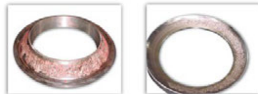
Circulating Water Pump bearing/race as found after APR notification of abnormal conditions
